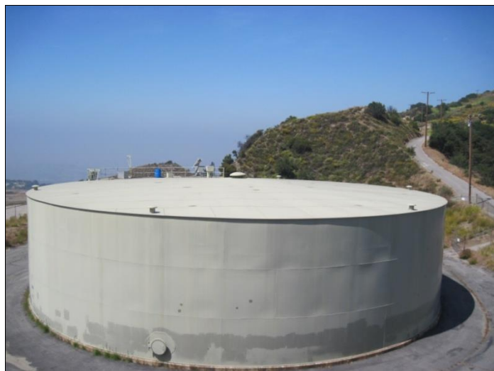
Figure 2-5: Example of a Recycled Water Storage Tank
