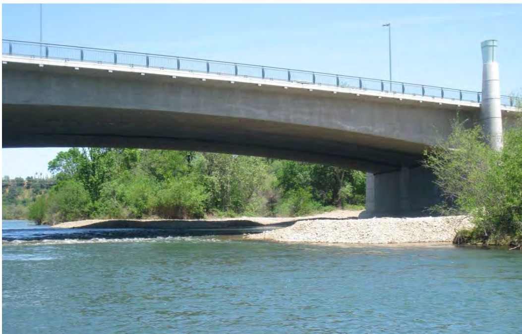
Figure A-14. Cypress Avenue Bridge North (Site 6) looking upstream across the river at the southeastern end of site.
