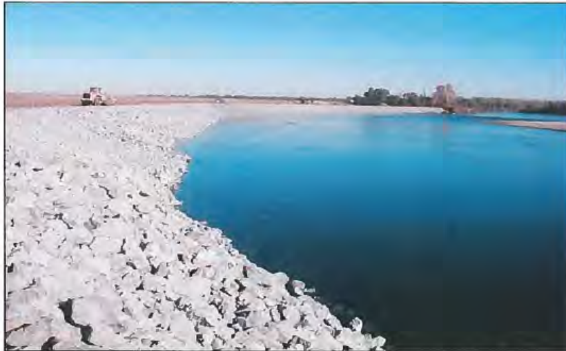
Figure 11. Agency revetment placed on an eroding bank on the middle Sacramento River under Executive Order S-01-06. Photo by Joe Silveira (USFWS), 2007.
