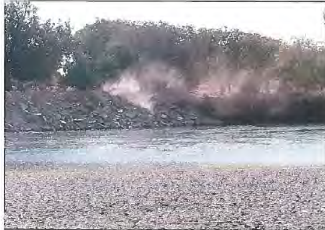
Figure 12. Private revetment being placed on an eroding bank on the middle Sacramento River. Photo by Dave Forwalter (DWR, Northern Region Office), 2007.
