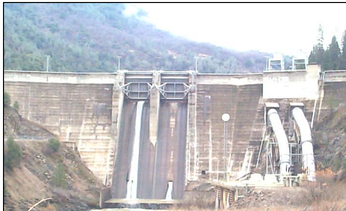
Figure 4-2. Pit 7 Dam, Located on the Pit River Upstream from Shasta Lake, is 200 Feet High
