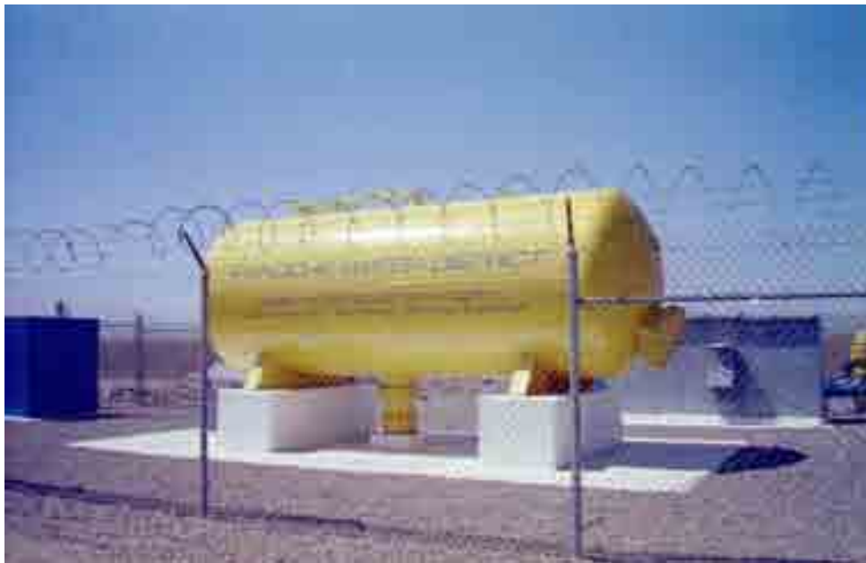
Figure 16-4 Drainwater Treatment Facility at Panoche Water District
