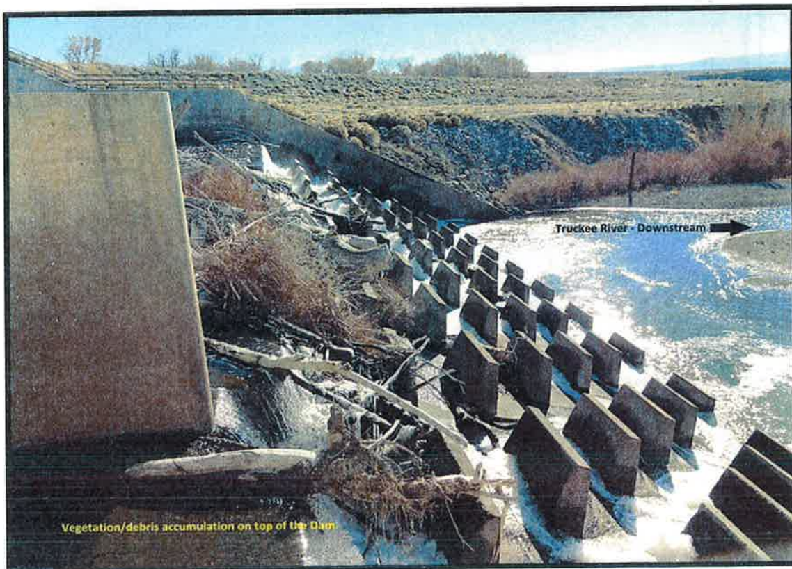
Figure 4 – Vegetation accumulation on Marble Bluff Dam
