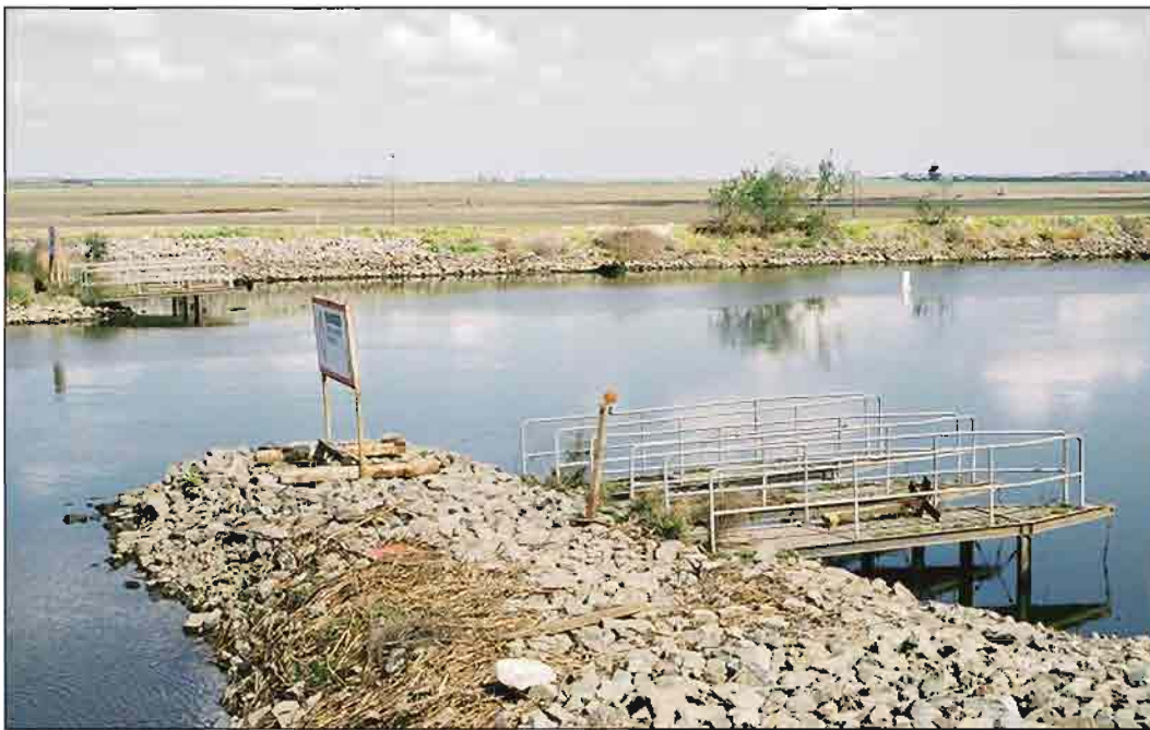
Photograph 7.6-6. Middle River Gate Site View is north of existing temporary rock barrier from the southern levee.
