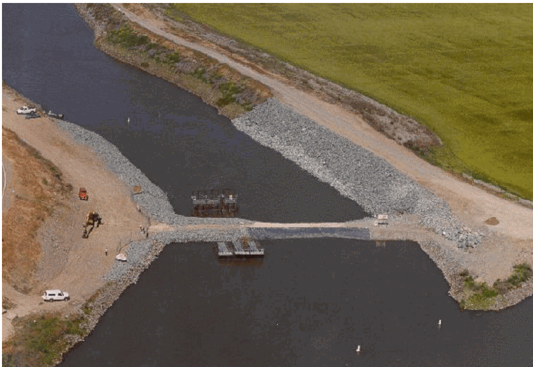
Photograph 5.2-22. Head of Old River Temporary Barrier with Culverts on Left Side that Allow Regulated Flow into Old River from the San Joaquin River (Source: California Department of Water Resources.)
