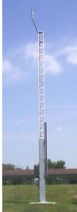
Figure 2-6: Example of a Radio Tower
