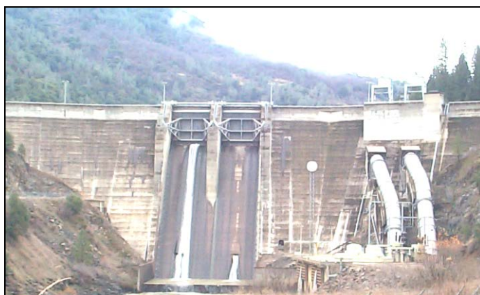
30 Figure 4-2. Pit 7 Dam, Located on the Pit River 31 Upstream from Shasta Lake, is 200 Feet High 32
