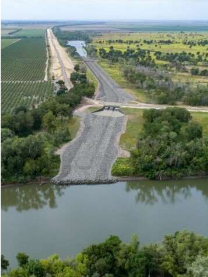
Figure 7. An aerial view of the progress made on the Fremont Weir gated notch in WY2022.
