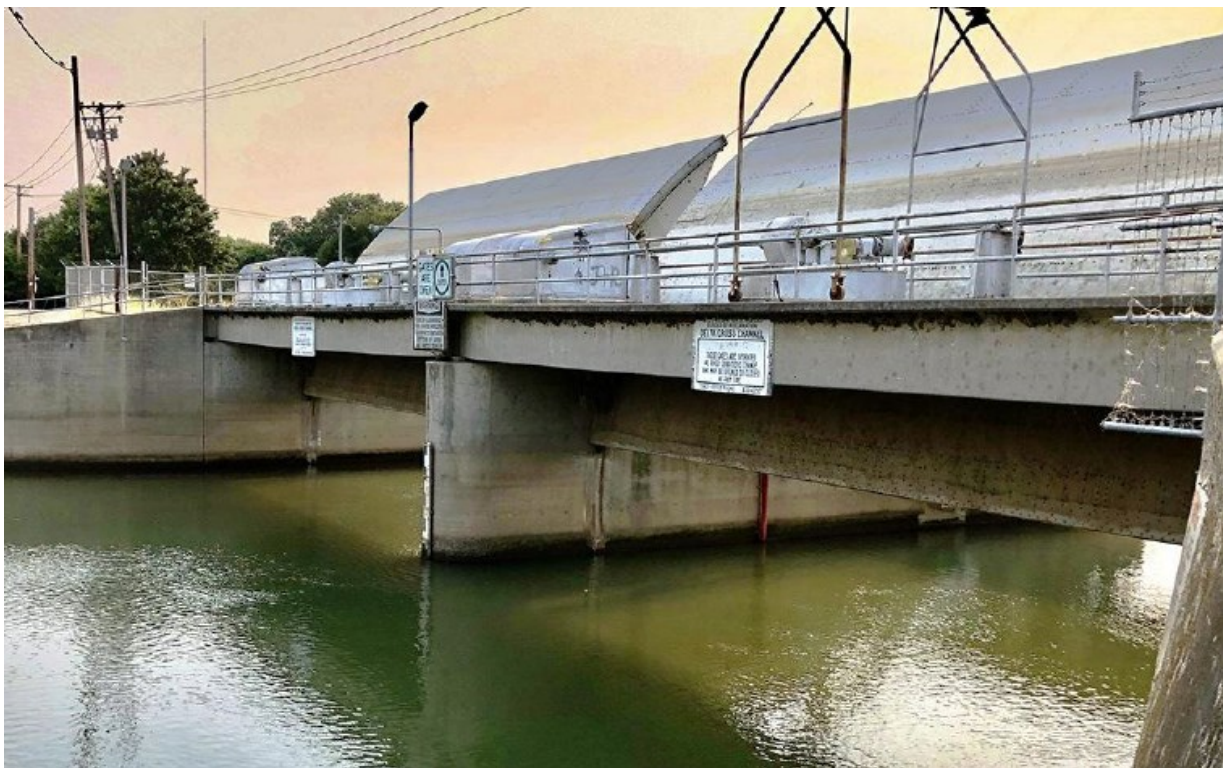
Figure 3. Delta Cross Channel Gates (Bureau of Reclamation/Todd Plain).
