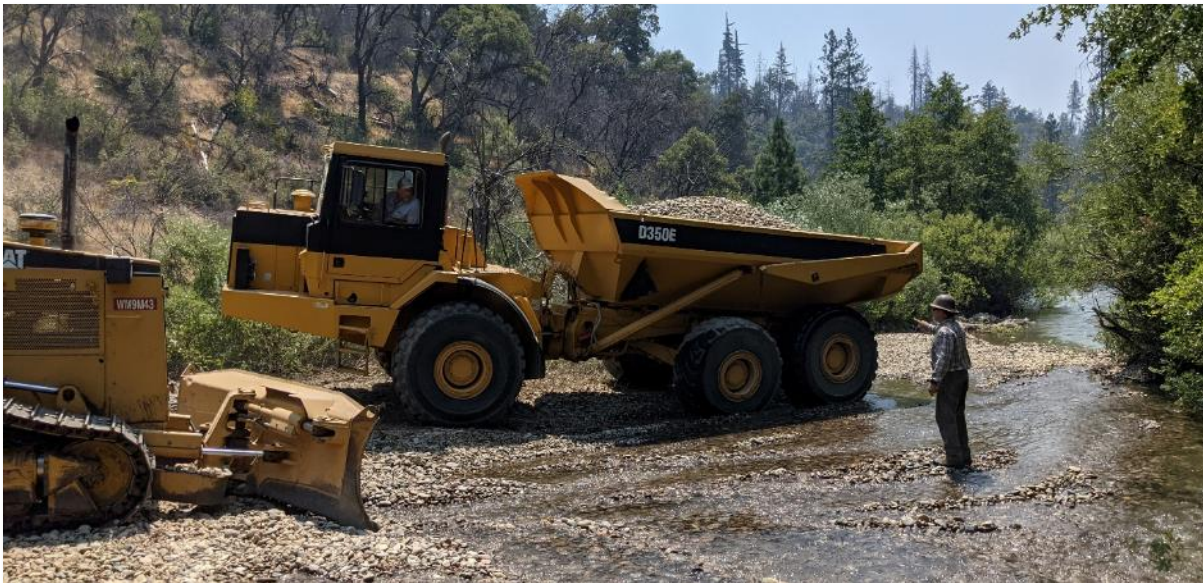
Figure 15. Implementation of the gravel augmentation project at the Below Dog Gulch site. Photo credit: Derek Rupert, Bureau of Reclamation.
