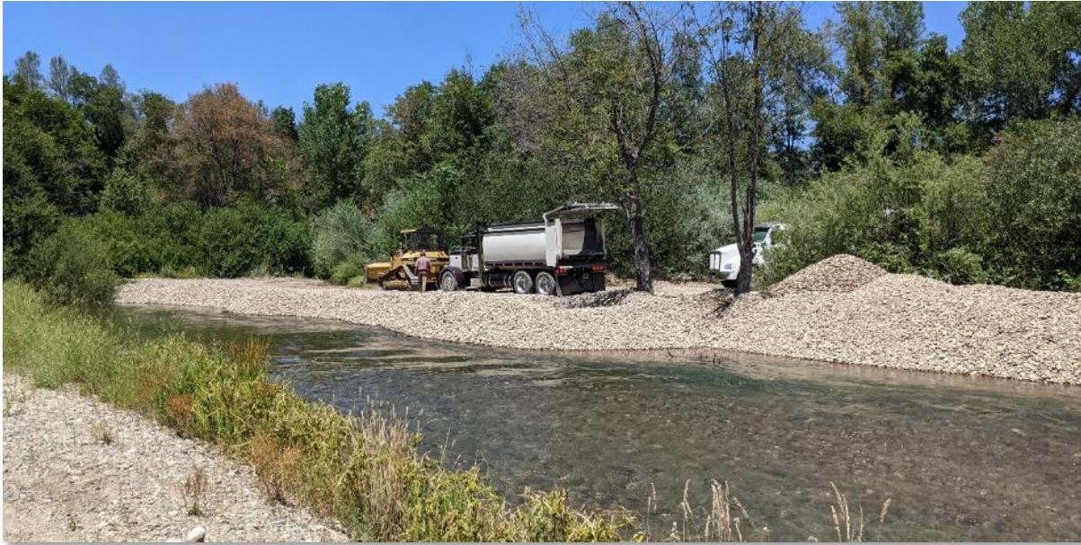
Figure 14. Construction of the lateral berm at the Above Phase 3A site. Photo credit: Derek Rupert, Bureau of Reclamation.
