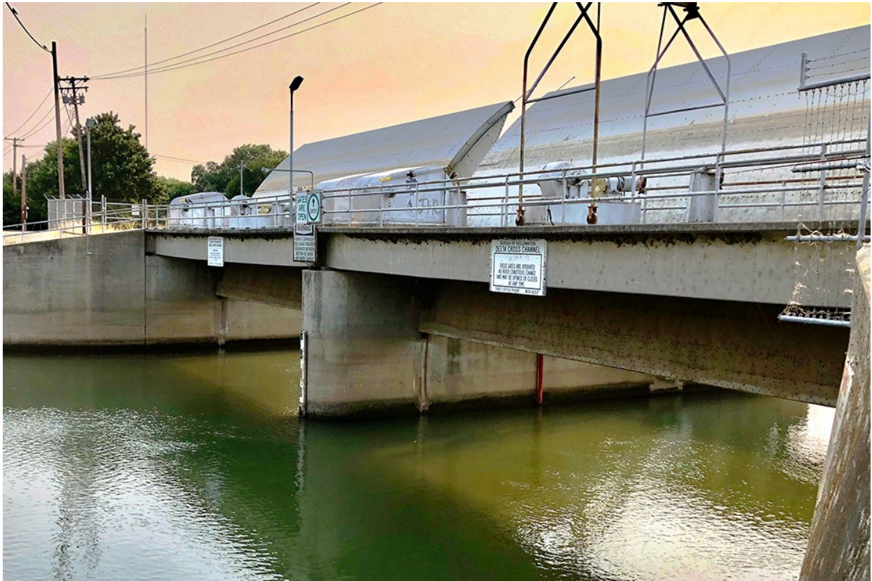
Figure 2. Delta Cross Channel Gates (Reclamation/Todd Plain).
