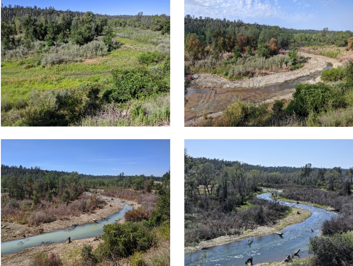
Figure 8. Top Left - A view of the upstream end of the project site showing the where the new channel will be constructed. Top right - A view of the upstream end of the project site showing the new channel being dug and prepared. Bottom left - A view of the upstream end of the project site showing the new channel with wood placement and its final morphology. Bottom right - A view of the upstream end of the project site showing the channel a few months after construction and following revegetation.
