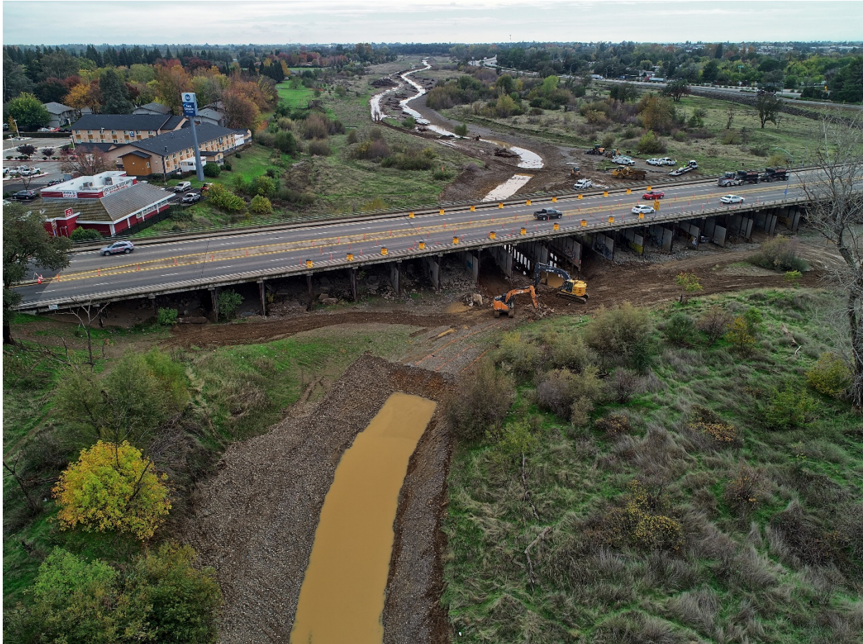
Figure 5. Looking downstream at the East Sand Slough project across the Highway 36 bridge with construction underway in November 2021.
