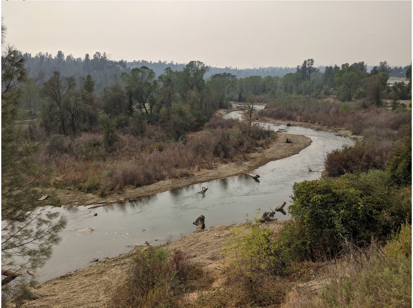
Figure 2. Newly constructed channel as part of Phase 3C. (Photo credit: Derek Rupert, Reclamation)
