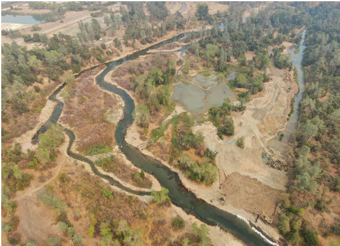
Figure 11. An aerial view of the Phase 3C project site during late-construction. Photograph credit: Aaron Martin (Yurok Design Team).
