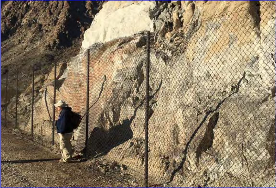
Photo 11. Proposed alignment of PBS barrier along the east-central portion of alignment (adjacent to the existing Coachella Branch of the All American Canal fence). View facing south.
