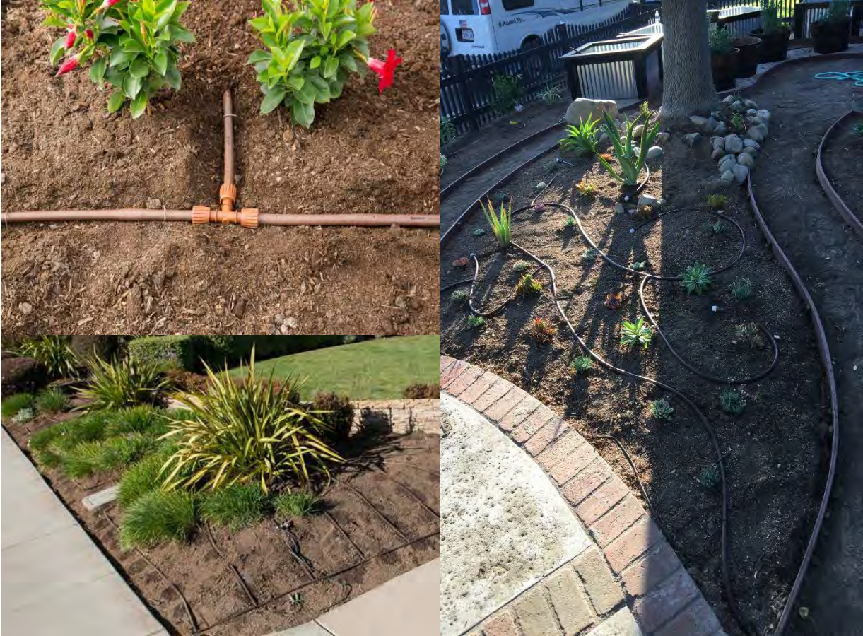
Figure 3. Examples of sites with drip irrigation installed.
