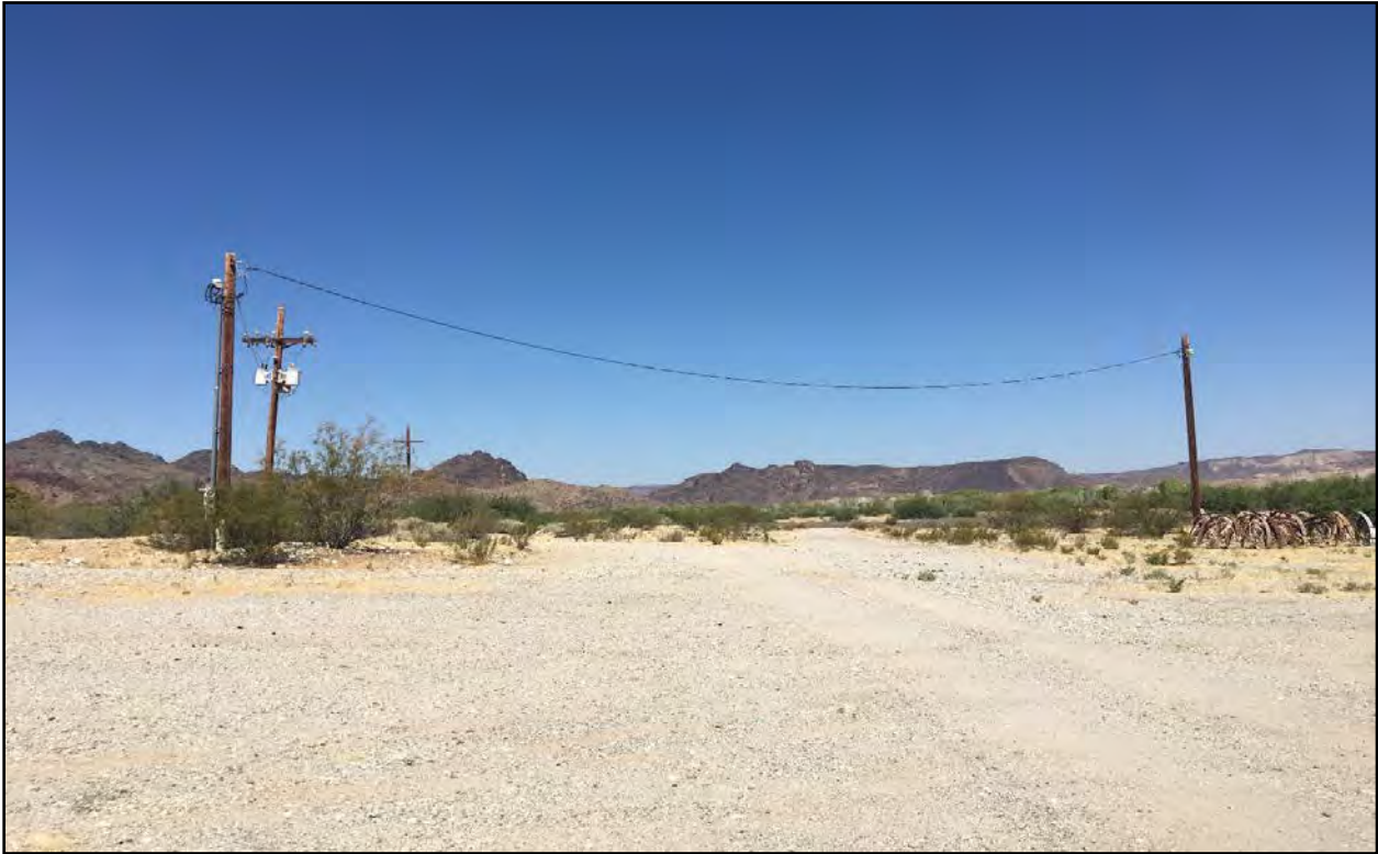
Figure 24. Planet Ranch Electrical Infrastructure (2017).
