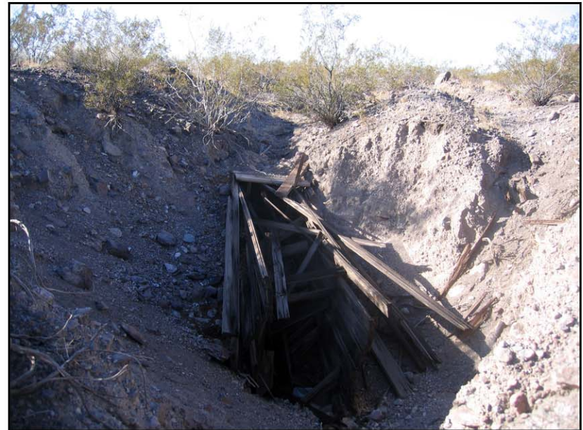
Photo 24 – Remains of subsurface wooden drainage, NE of mill site, facing W. January 9, 2007.
