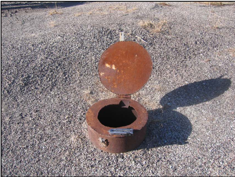
Photo 31 – Test well showing vandalized well completion. NE of mill site. January 9, 2007.
