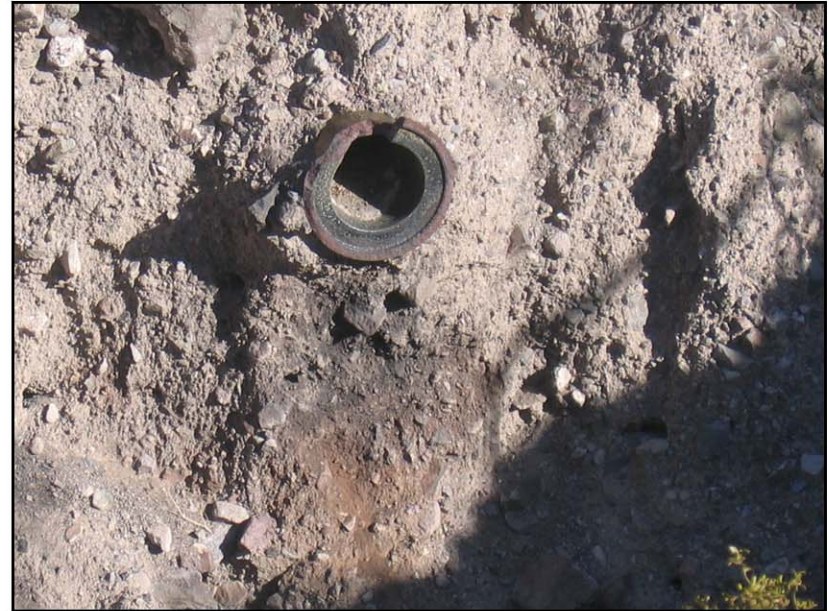
Photo 22 – Exposed pipeline, NE of mill site. January 9, 2007.
