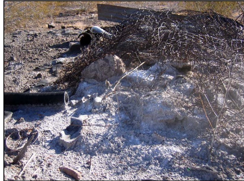
Photo 34 – Weathered apparent friable asbestos in mill site E of former calcining kilns. January 9, 2007.
