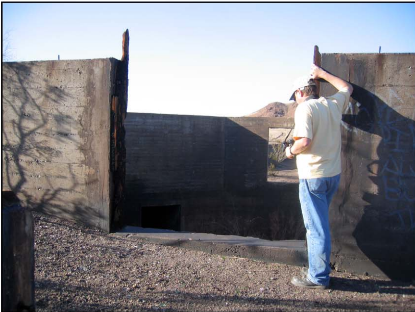
Photo 19 – East octagonal sump depicting fall hazard facing NW. January 9, 2007.
