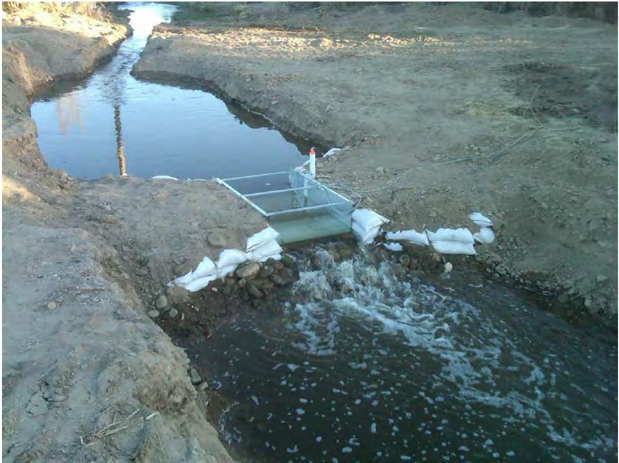
Photo 5. – 10 cfs Maximum Capacity Non-Adjustable EF10 Galvanized Steel Nuway “EZ Flow” and Stilling Well with Locking Cap.
