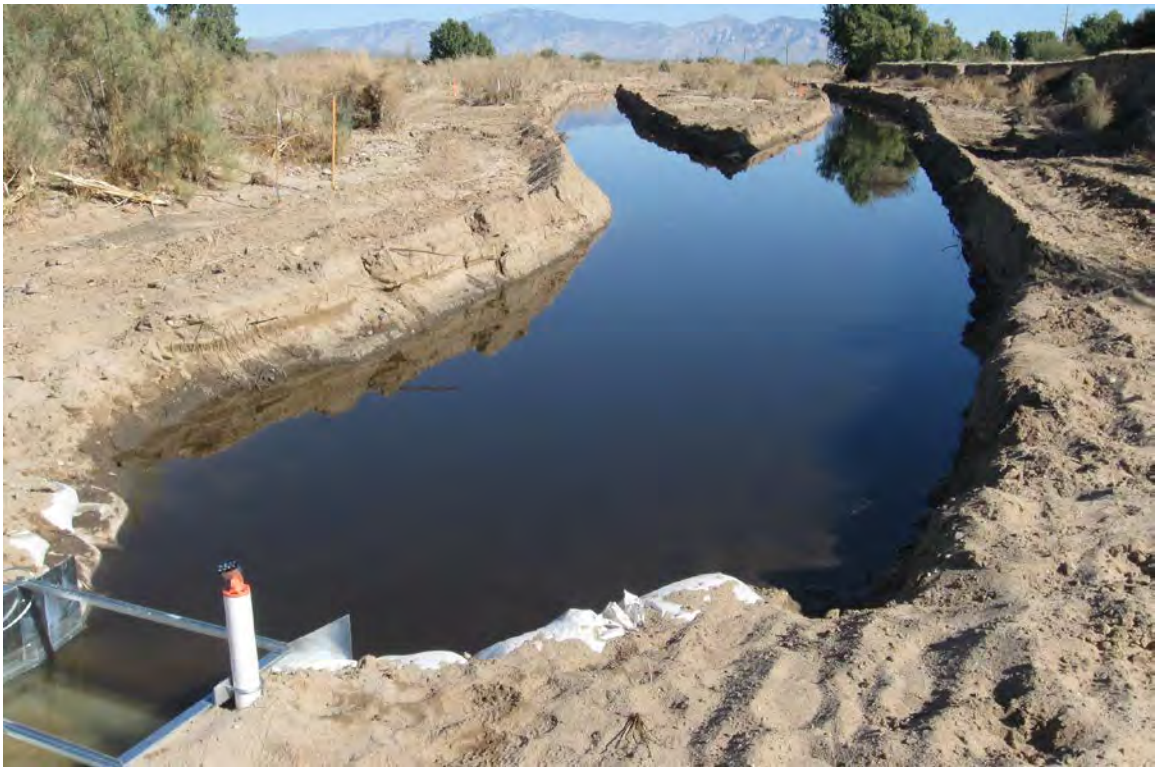
Photo 10. – Looking Upstream at the Dirt Berm Barrier that was Breached at the Convergence of Channels 1 and 2.
