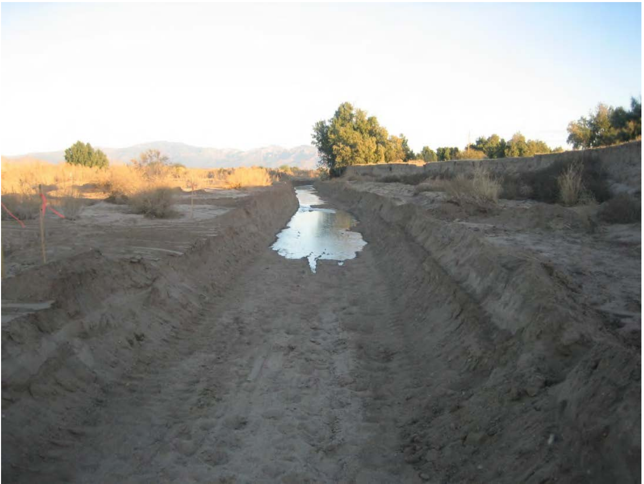
Photo 8. – Water First Diverted to ERDP on January 28, 2011. Note fines on bottom of Channel 1.
