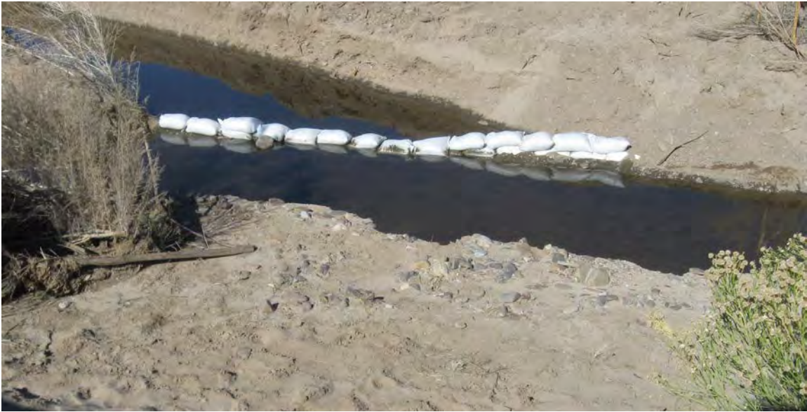
Photo 9. – Sandbag and Dirt Berm Barrier Breached at Divergence of Channels 1 and 2.
