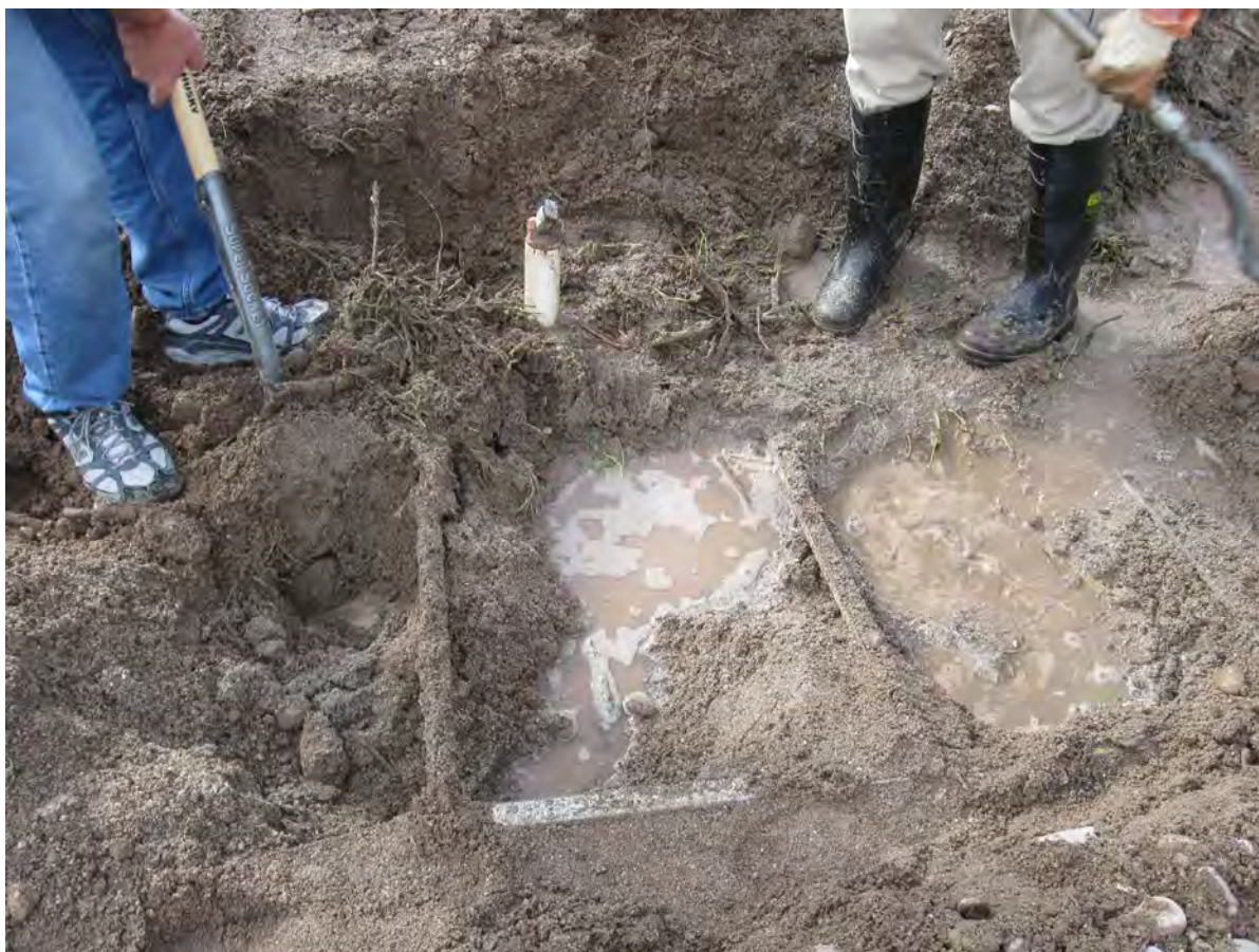
Photo 17. – Buried Upstream Flume after July 5 th and 6 th Stormflows.
