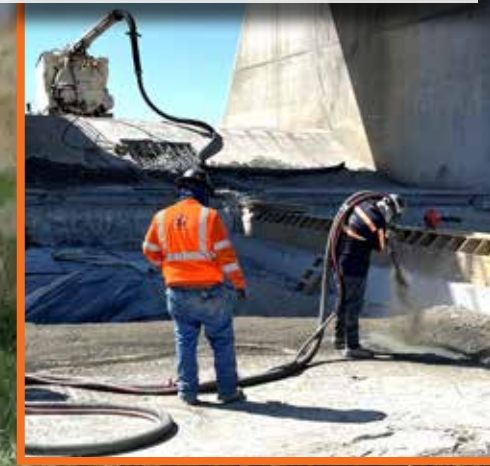
Contract employees from Harrison Western immediately apply shotcrete to approved foundation rock to protect the foundation before placing a sand and gravel filter. Certain rock types such as pictured here can deteriorate or slake upon exposure to the elements.
