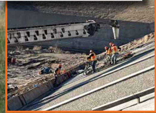
Contractors place a mud mat over properly graded sand and gravel filter material prior to installing the anchor bar. The sand and gravel filter underlies the spillway slab and is a critical feature of any spillway. A properly designed and installed filter prevents failures from occurring and can be used as a warning system if fine grain material is seen exiting the filter.
