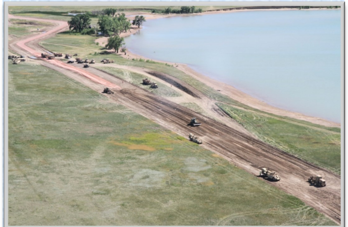
(Above) South Dakota Army National Guard troops constructing Bird Island View Road.
