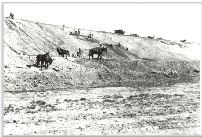
(Above) Shaping the slope of the upstream face of Belle Fourche Dam as a foundation for the pavers, May 15, 1909.
