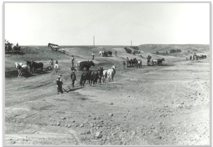
(Above) The above photograph was captured during construction of Belle Fourche Dam's main Inlet Canal at Station 110 on August 22, 1905.
