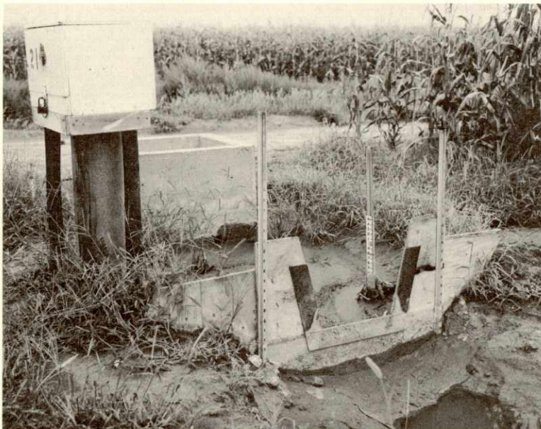
Standard 1.5-foot Cipoletti weir and recorder, water use study, Frenchman- Cambridge Division
