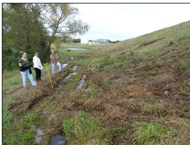
Figs. 1 and 2: Stigler Lake Dam. Top: The earthen dam and reservoir on the left. Bottom: The downstream dam face showing seepage.
