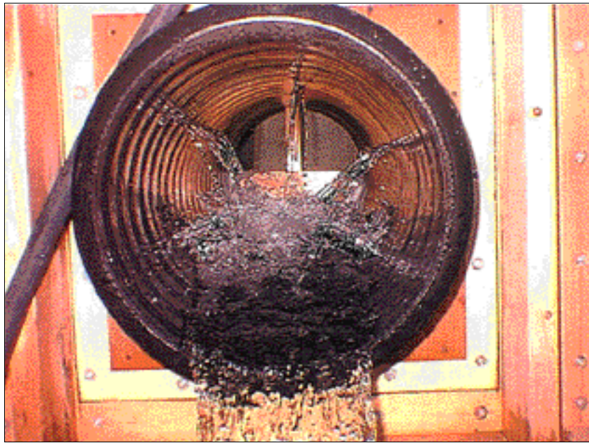
Figure 10 – All the 5/16-inch diameter perforations are abundantly flowing water. Flow rate is approximately 56 gpm (23 gpm per linear foot of drain pipe).
