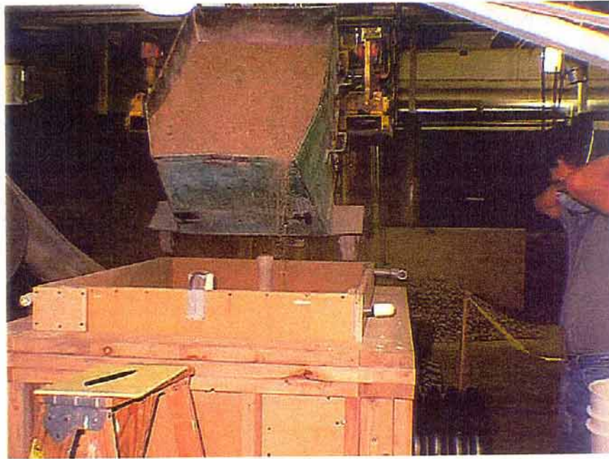
Figure 6 - Special forklift used to dump “boats” of sand envelope into pipe box.
