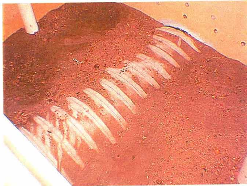
Figure 7 - View of pipe box interior with partial backfill. Length of drain pipe covered with geotextile is 28.8 inches. The 2-inch PVC standpipes deliver water to the PVC well-screen distribution network around the inside bottom perimeter of the pipe box.
