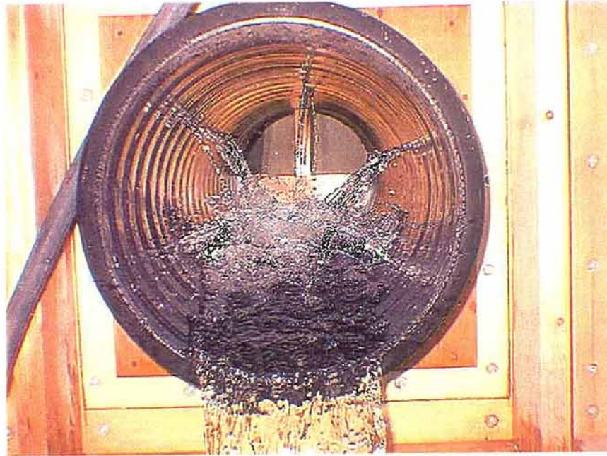
Figure 9 - All the 5/16-inch diameter perforations are abundantly flowing water. Flow rate is approximately 56 gpm (23 gpm per linear foot of drain pipe).
