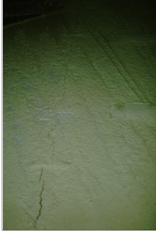
A view of the shrinkage crack in the first Koyna model.
