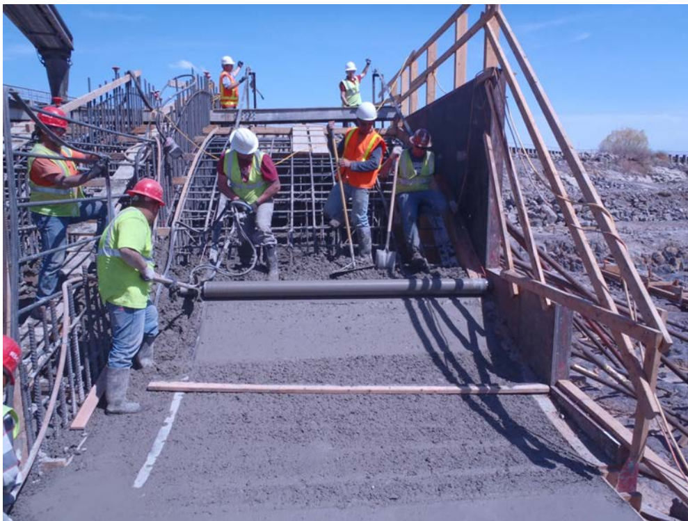
Figure 2 – Photograph showing field fabricated tools and methods used while forming an ogee crest at Minidoka Dam.
