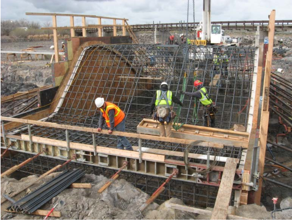
Figure 1 – Photograph showing construction workers placing reinforcement and formwork for an ogee crest at Minidoka Dam.
