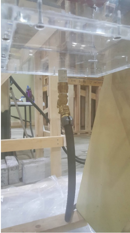
Figure 5. Hose attached to shut-off valve at bottom of tank.
