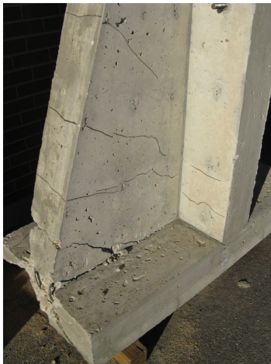
Figure 23. – Actual damage to counterforted wall.
