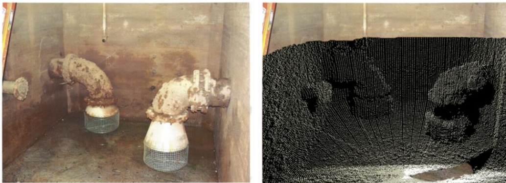
Figure 3.—Left – Photograph of a pump sump in Reclamation's hydraulics lab in Denver, Colorado. Right – 3-D point cloud of the water-filled sump (over 100,000 profile points) overlaid on the photograph.
