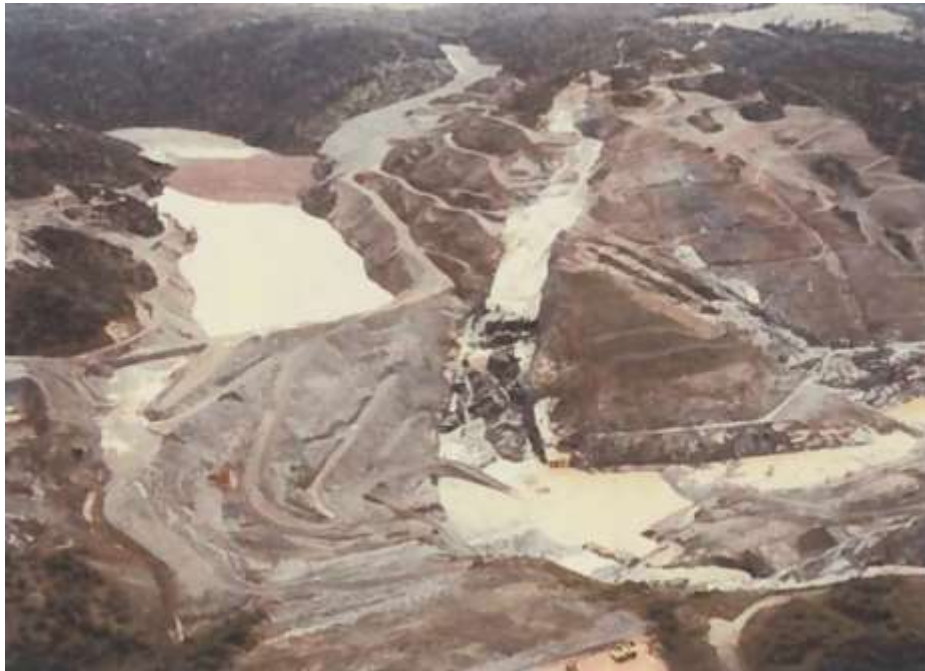
Figure A5. Aerial photo of the downstream face of cofferdam and foundation excavation during large flood event. The fuse dike and the long buttress fill channel downstream of the fuse dike can be seen to the left of the cofferdam.
