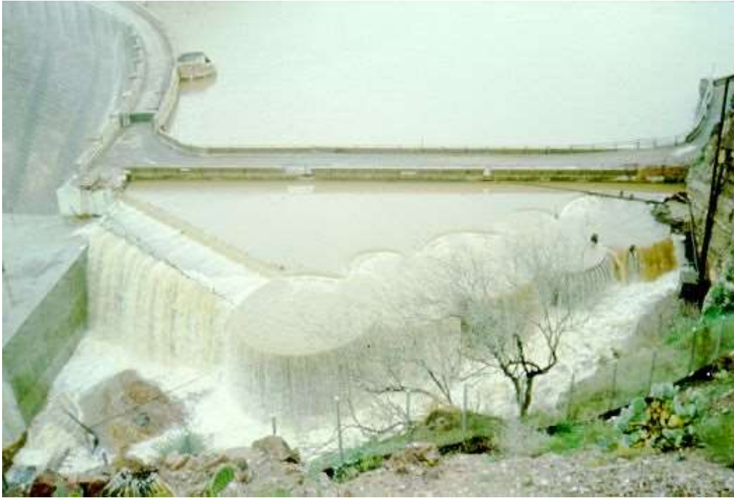
Figure 6. Aerial view of cellular cofferdams being overtopped in 1993.
