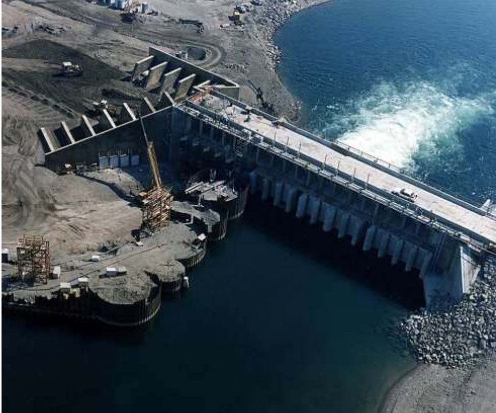
Figure 12. Aerial view of cellular cofferdam upstream of Jackson Lake Dam during the second stage of construction.
