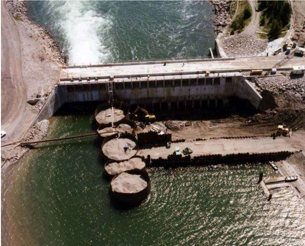
Figure 11. Aerial view of cellular cofferdam upstream of Jackson Lake Dam during the first stage of construction after July 10.
