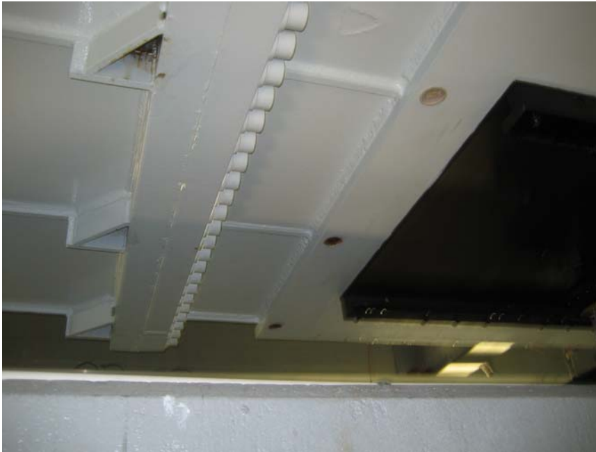
Photo 21. Structural bolted connection of LHPOST shake table platen connection—typical of two connections.
