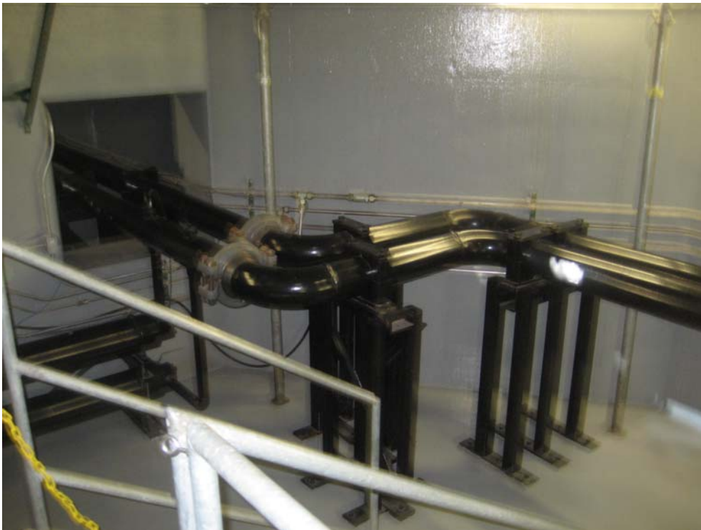
Photo 24. Primary hydraulic fluid delivery pipes.
