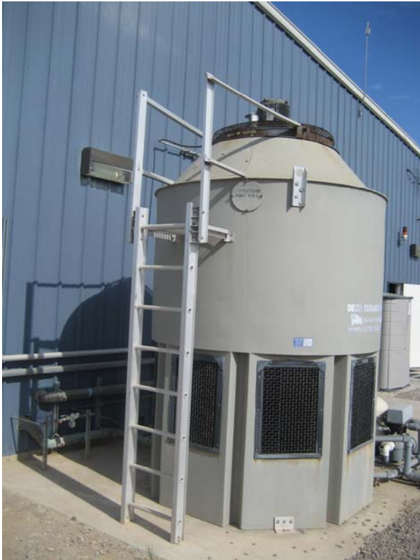
Photo 25. Coolant tank for LHPOST hydraulic system.
