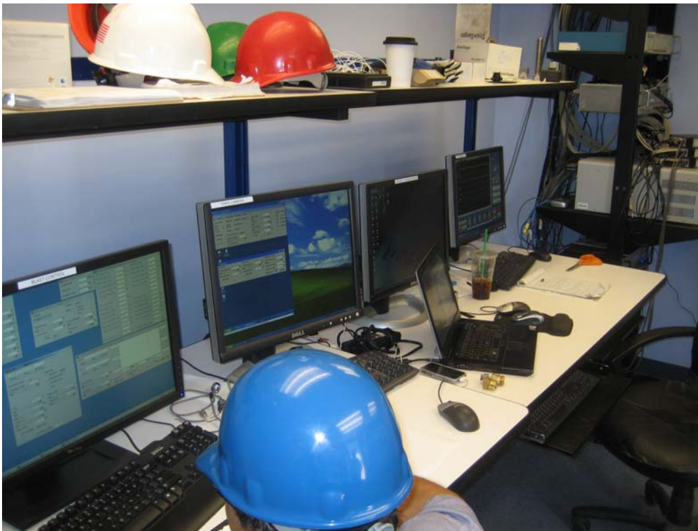
Photo 28. Client workstation for primary data acquisition servers.
