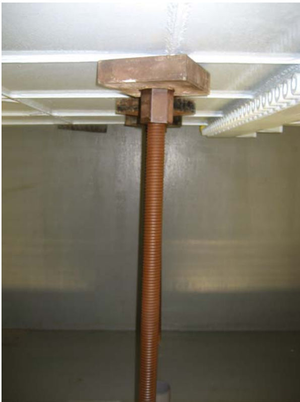
Photo 22. Close-up of threaded post-tensioned anchor for pier foundation being constructed on top of LHPOST table—see Photo 4.
