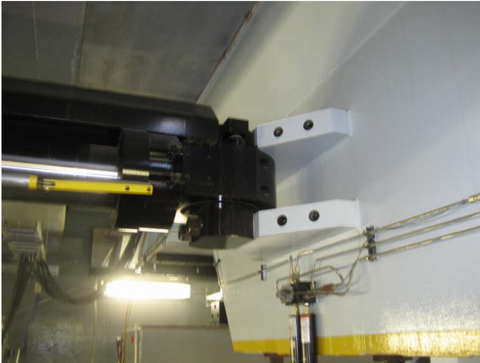
Photo 23. Hydraulic actuator pin connection to LHPOST shake table.
