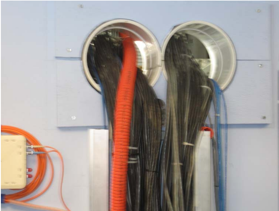
Photo 27. Data cables from LHPOST instrumentation to collection servers—see Photo 26.
