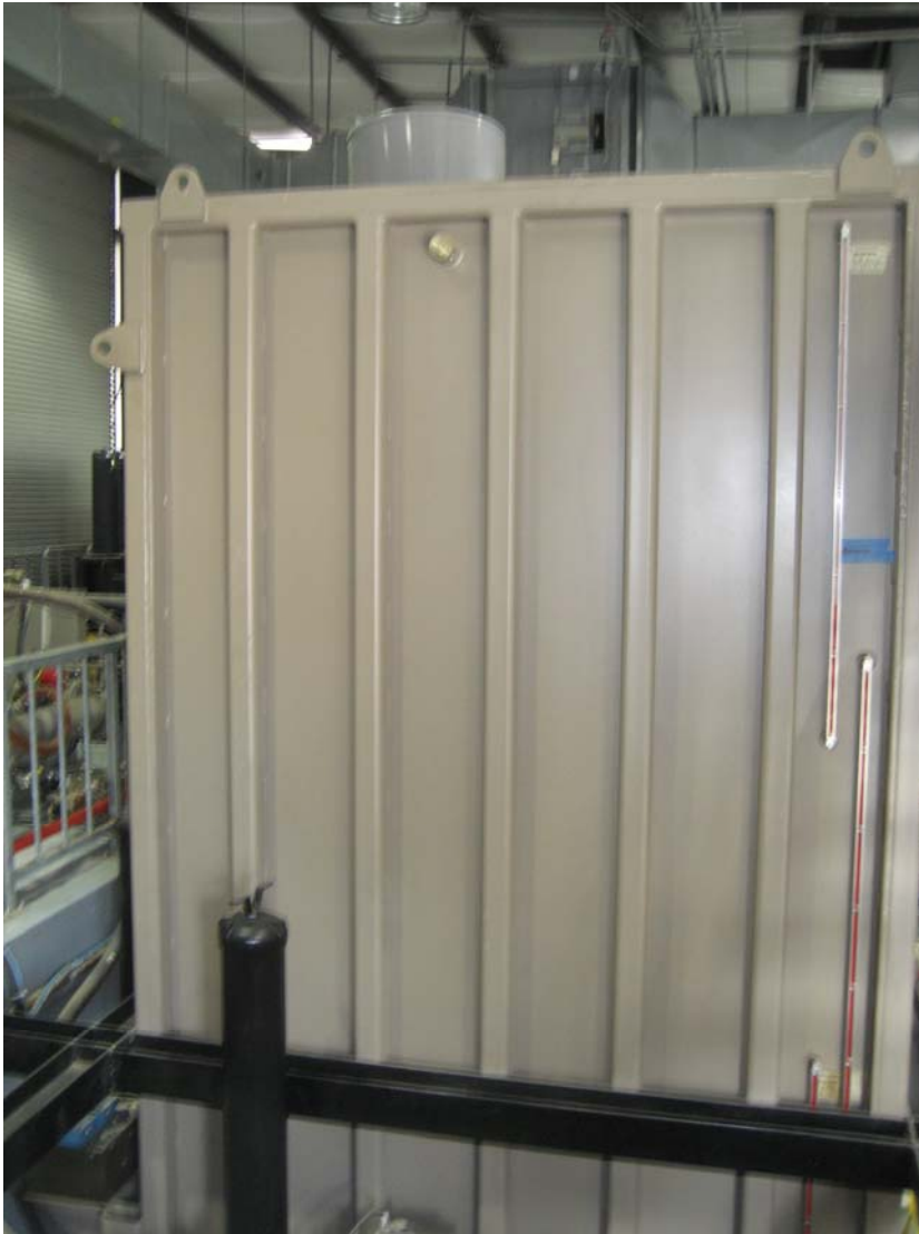
Photo 16. Oil tank for LHPOST hydraulic system.
