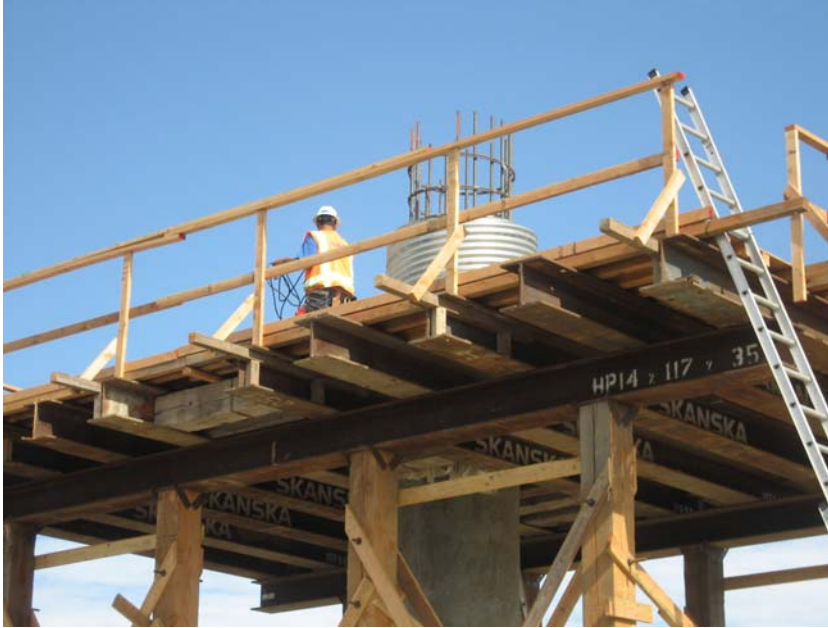
Photo 5. Reinforcement cage extending from construction joint of bridge pier being construction on LHPOST shake table.
