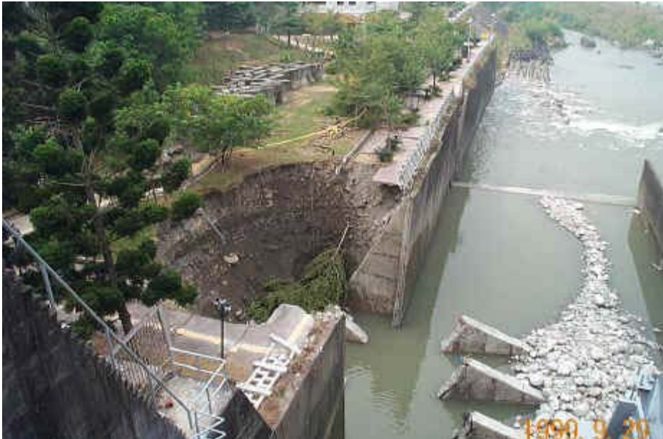
Figure 7. —Failed spillway wall at Shih-Kang Dam.
