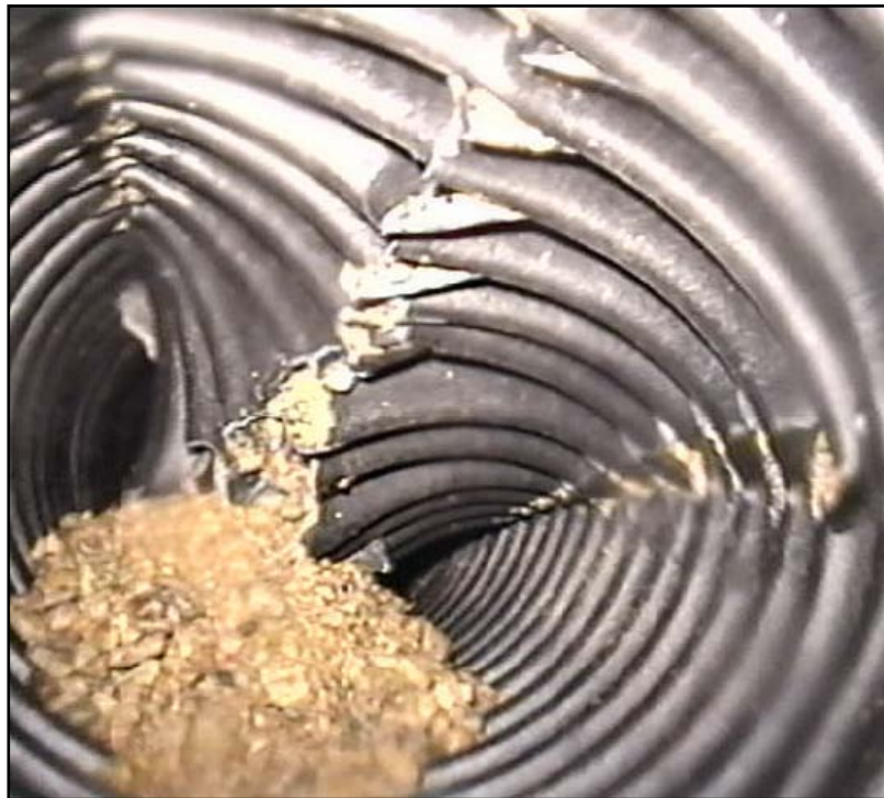
Figure 1-1.—Collapse of corrugated plastic pipe toe drain.
