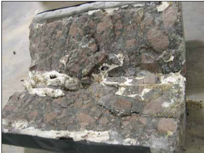
Figure 10. —Sand grains embedded in crack after injection; paste has washed out at reduced dosage of anti-washout admixture.
