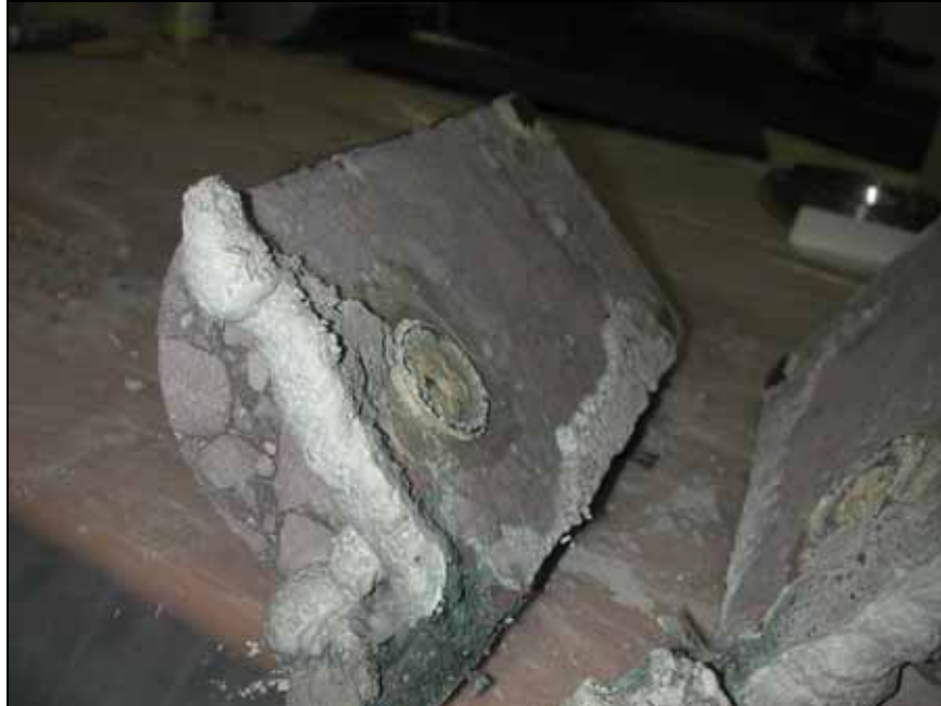
Figure 14. —End view of 6-mm ( \frac{1}{4} -in) wide crack test specimen after test filling with 100-L/min (25-gal/min) crack flow.
