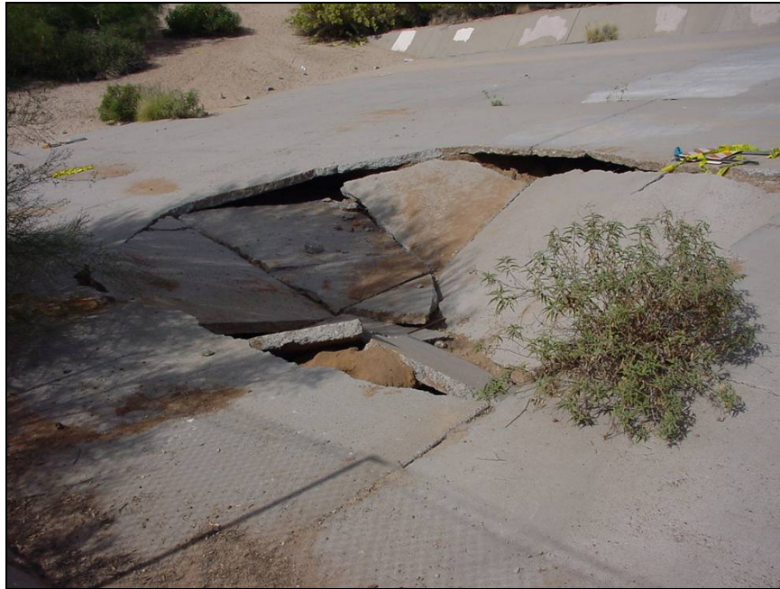
Figure 4. —Structural collapse of the slab system occurs when enough undermining has occurred to cause loss of support. This damage is typical of slabs placed on soil foundations (note: this slab is not reinforced so failure is more evident).
