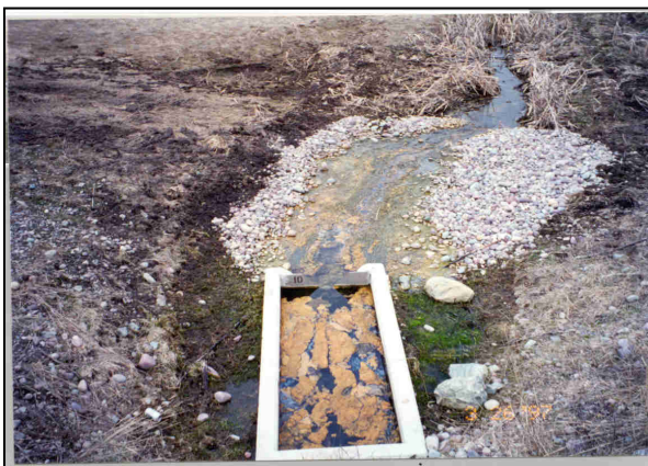
Figure 5. —The weir shows an example of biofouling.
