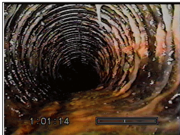
Figure 6. —The bacterial growth is partially covering the inside of 8-inch diameter HDPE pipe.
