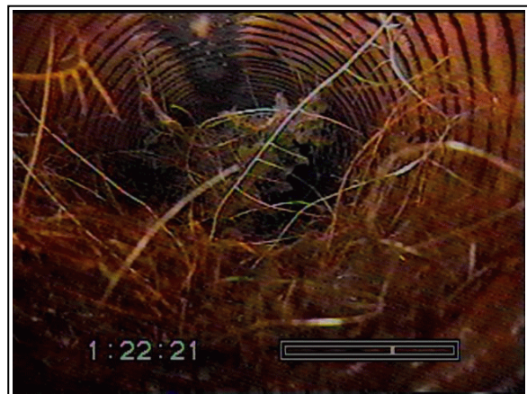
Figure 12. —Vegetative growth shown fouling 8-inch diameter HDPE pipe.
