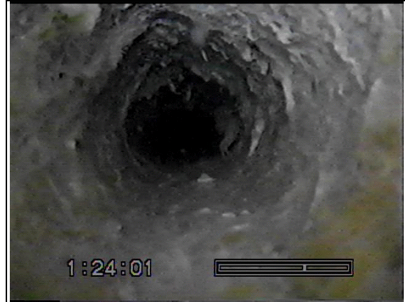
Figure 8. —Bacterial grow is shown completely covering the 8-inch diameter HDPE pipe.
