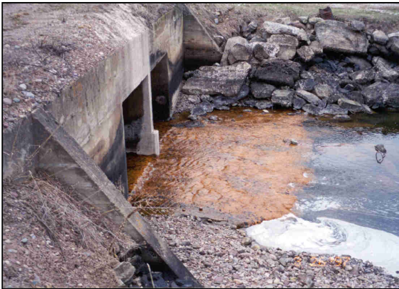
Figure 3. —The outlet shows an example of biofouling.
