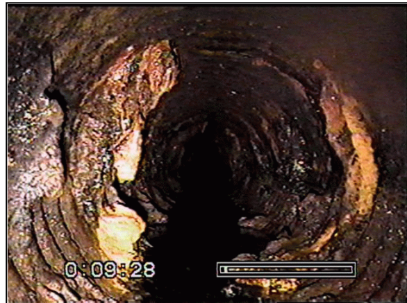
Figure 10. —Calcium carbonate precipitate was observed covering the 18-inch pipe interior about 60 ft upstream of the outfall exit portal of a toe drain.
