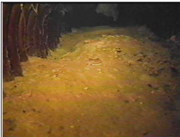
Figure 11. —Sediments were observed fouling the invert portion of a 12-inch diameter HDPE pipe.
