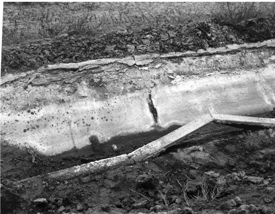
Figure 6.—Deterioration of concrete canal lining caused by sulfate attack. Note that deterioration is greatest in the saturation zone because of high groundwater sulfate concentrations.
