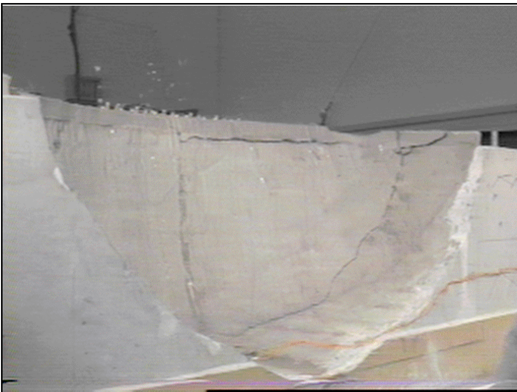
Figure 30b.—Model 11 - vertical joint south view, initial cracking.
