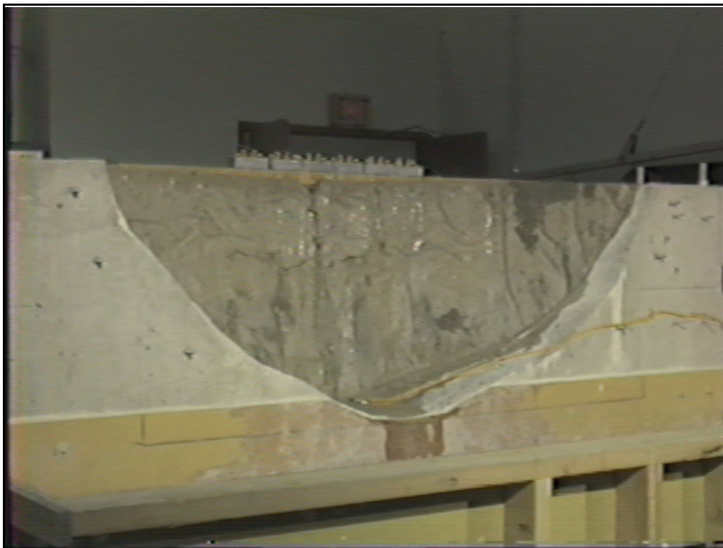
Figure 31a.—Model 15 - 17x2 joints, initial cracks.
