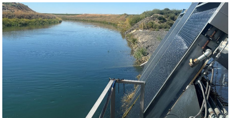
DS&I field visit to Warden pumping plant, Columbia Basin Project, Washington, August 28, 2024.
