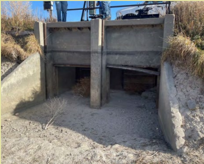
Sediment buildup at lateral entrance gate.
