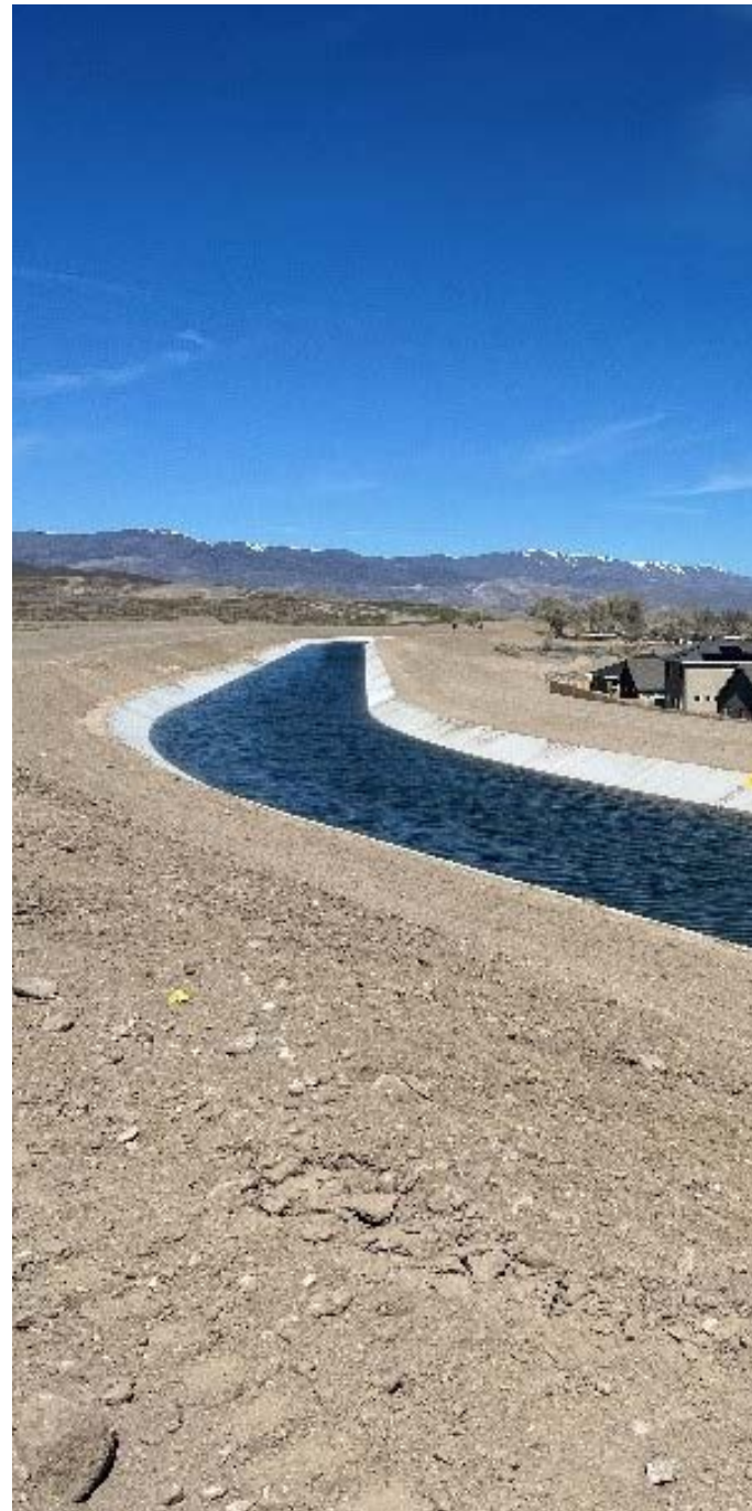
Truckee Canal Public Safety Improvement Project Phase I construction, which began in November 2022, was announced as complete on May 22, 2024.
