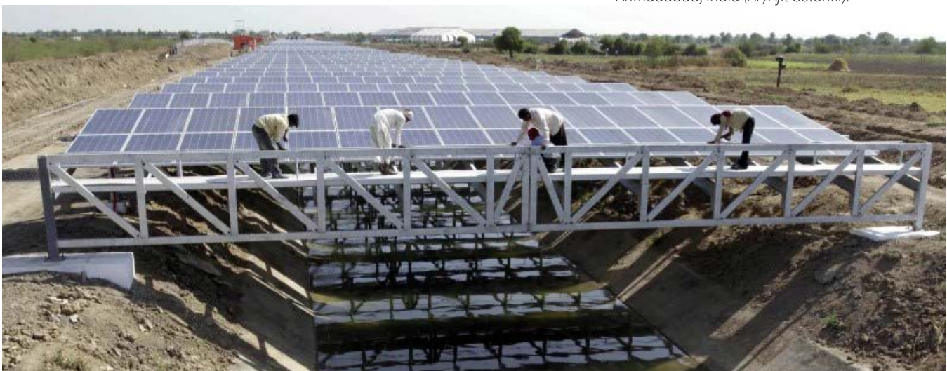
Workers installing solar panels covering the Narmada Canal at Chandrasan village, outside Ahmadabad, India (AP/Ajit Solanki).
