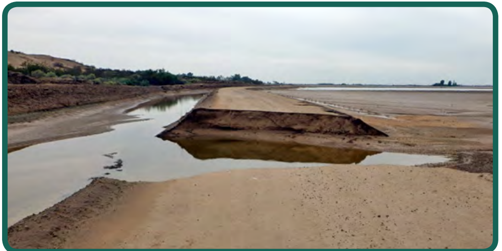
Facing southerly observing a breach in the East Main Canal embankment about ½ mile downstream of the Yuma County Water Users' Association Headquarters near County 15 th Street and Avenue C in Somerton, Arizona. Sediment, storm and canal waters flowed into agricultural fields to the right (west).
