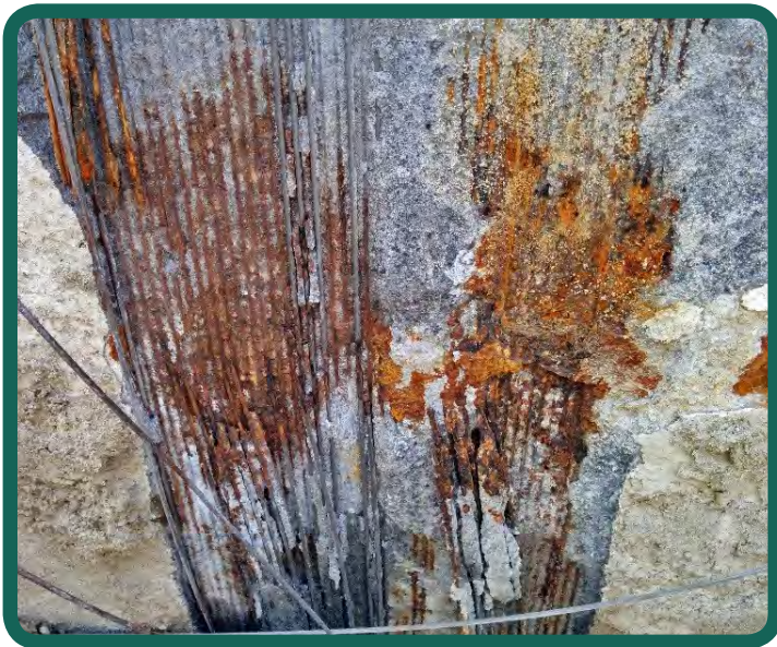
Corroded wires on PCCP.
