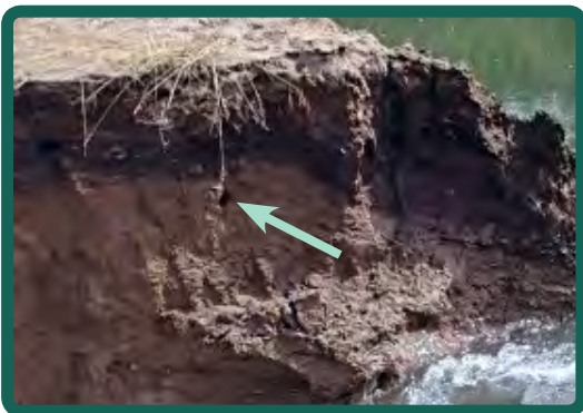
View of the breach from the crest of the canal embankment. A 2 to 3-inch rodent hole was noticed on the right side of the breach.
