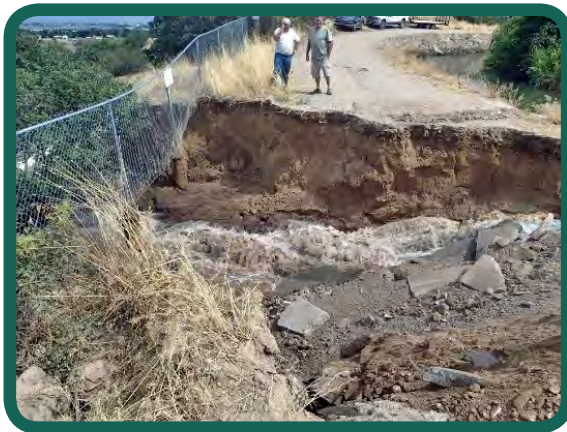
View of the breach from the crest of the canal embankment. 12:02 pm, August 25, 2015. Note the large pieces of concrete used to stop the flow out of the breach.
