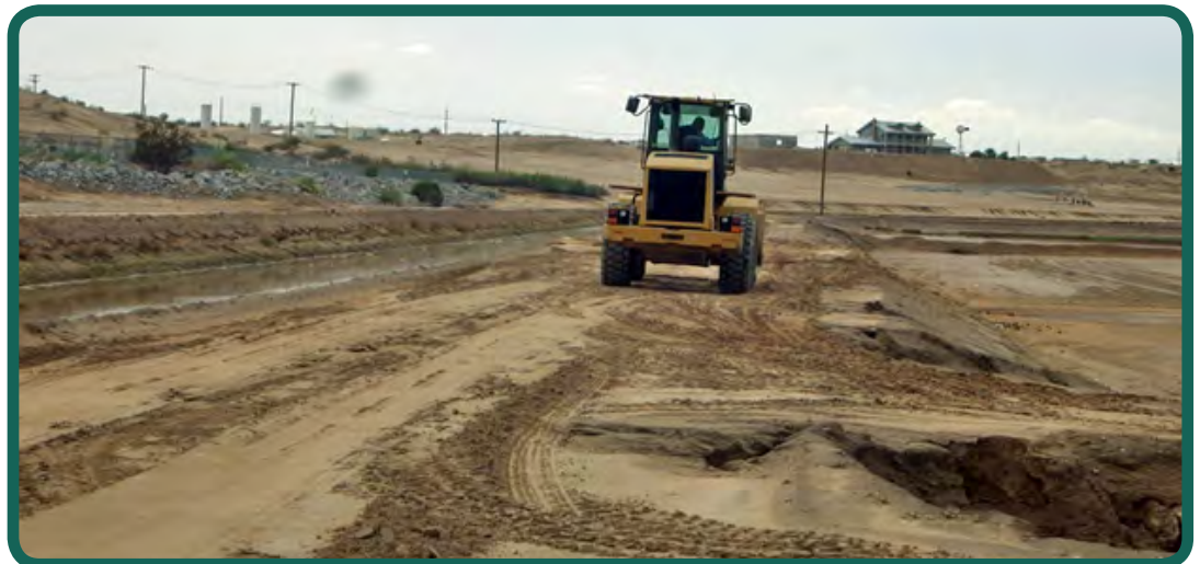
Facing southerly observing YCWUA O&M personnel repairing a breach in the East Main Canal on September 9, 2015, the day after the storm event occurred.
