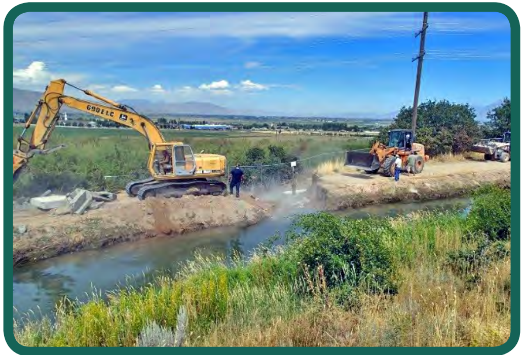
View of the breach from the uphill side of the canal, 12:06 pm, August 25, 2015.
